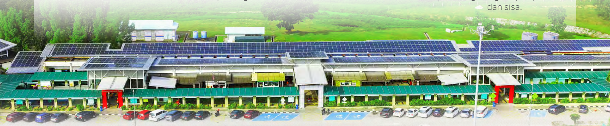
PLUS Malaysia - Harnessing renewable energy through a solar PV system, with 12 solar panels installed at RSA Dengkil Northbound.
